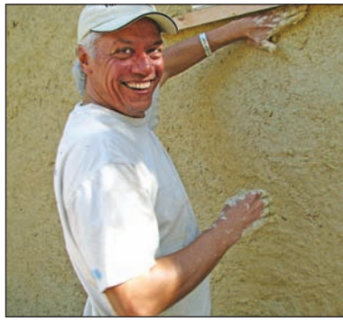
Austin architect Ben Obregon applies earth-plaster to exterior of straw bale wall.
