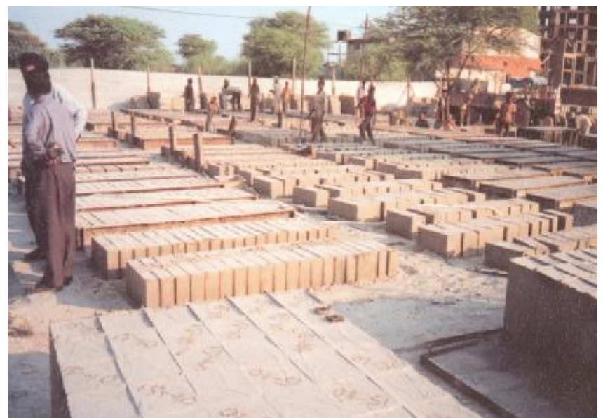
Demolding of blocks the day after casting or earlier it accelerated by either steam, heat or chemicals.
