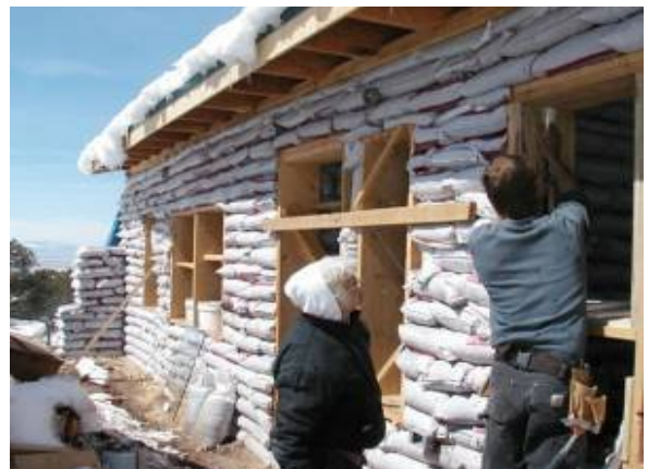
Above: Earthbags are built by stacking, with conventional doors and windows between.
